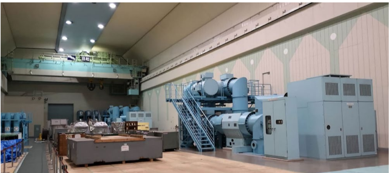
Figure 5-14 | Application of variable-speed units for Komarukawa pumped storage power station in Japan
